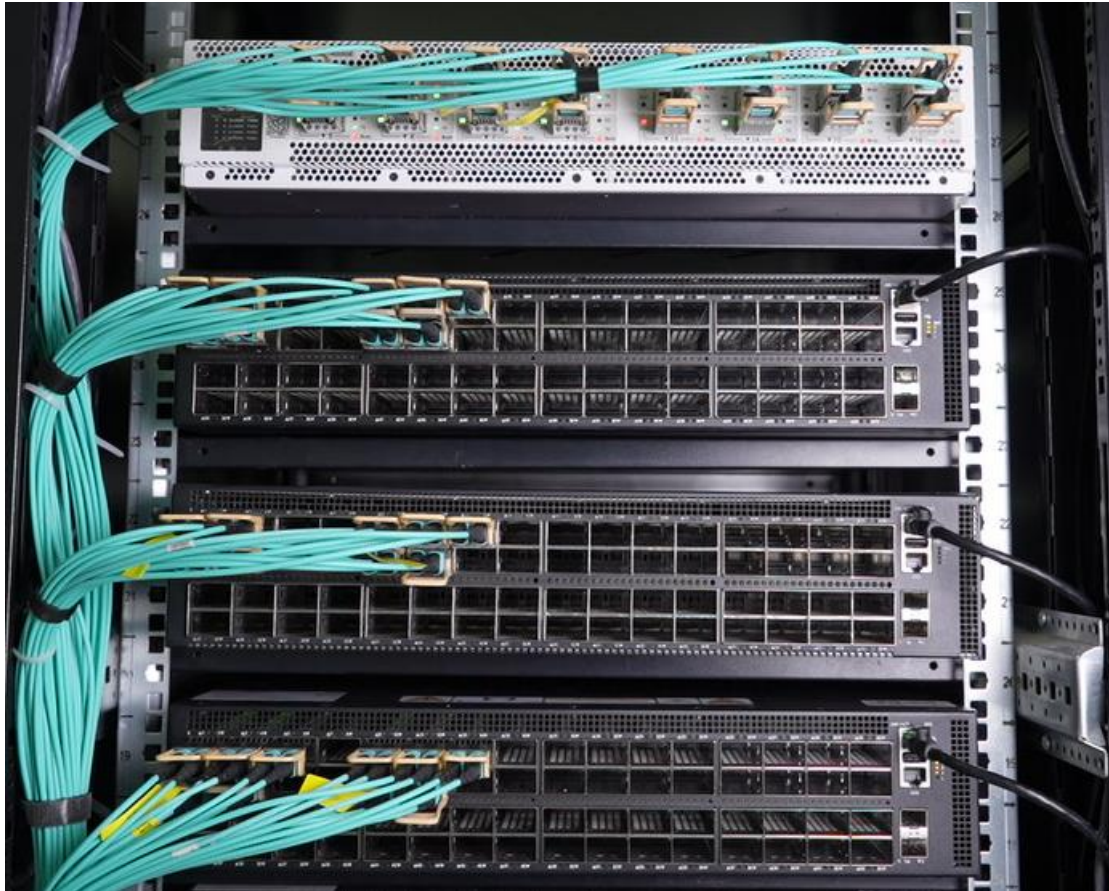
Picture 2-1 Physical Wiring Environment
